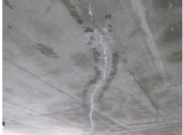
Crack on ceiling
