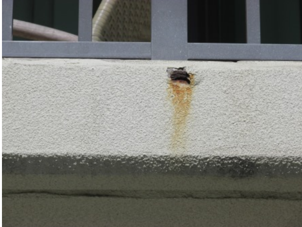
Exposed reinforcement at balcony edge
