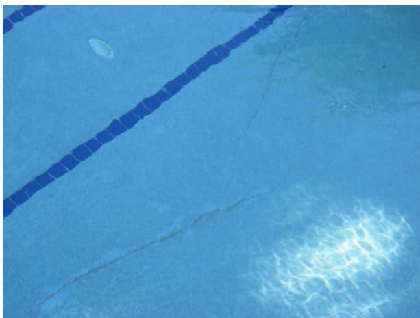
Lazy river plaster cracks
