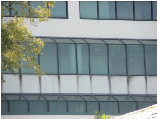
Stucco paint finish biological growth
