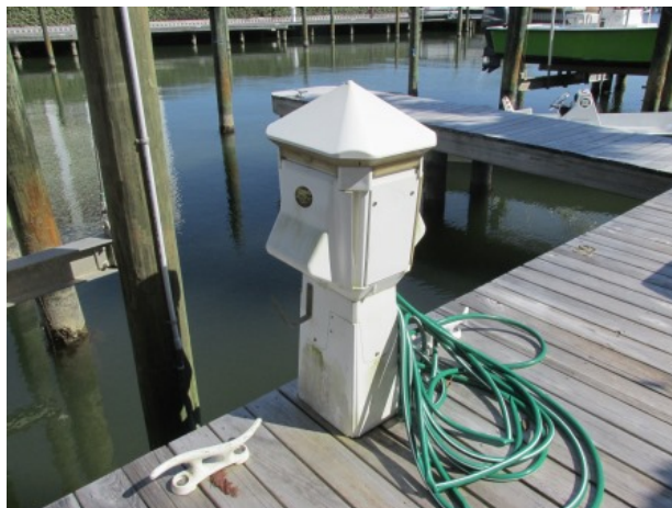
Typical power pedestal
