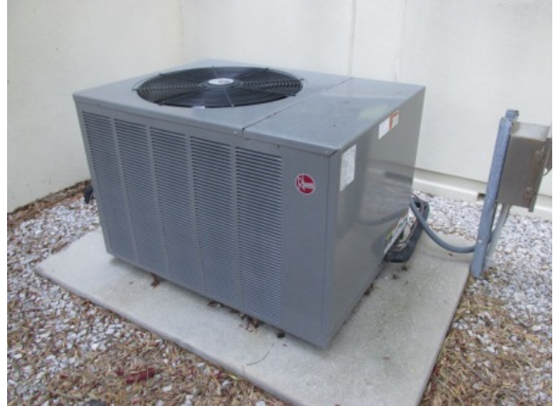
Split system condensing unit
