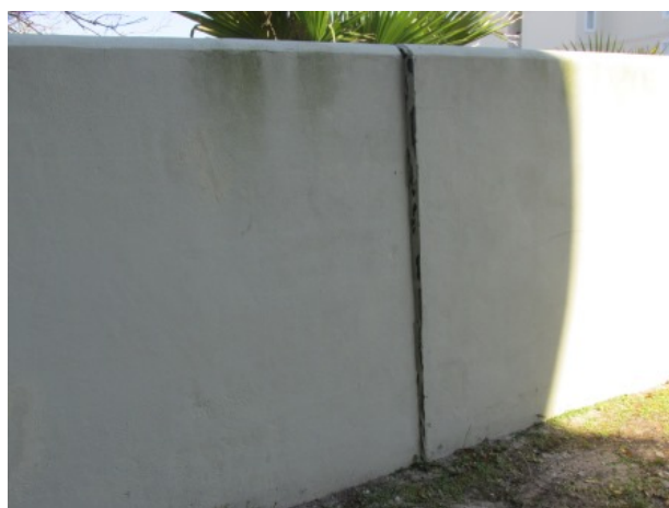
Settled perimeter wall section
