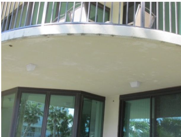
Balcony finish deterioration
