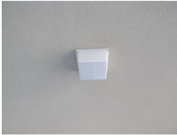
Breezeway light fixture
