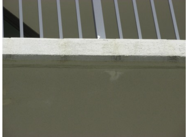
Balcony finish deterioration
