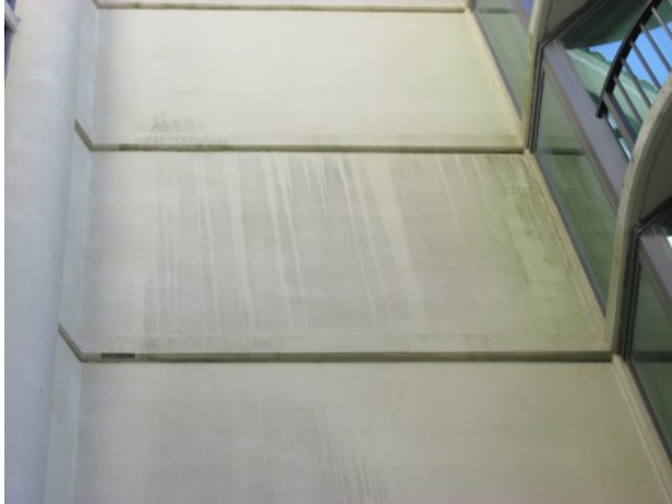
Stucco paint finish biological growth
