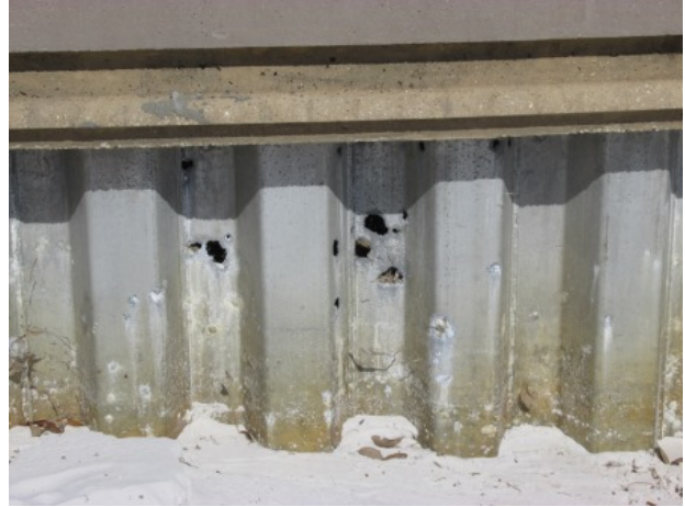
Holes in steel bulkhead
