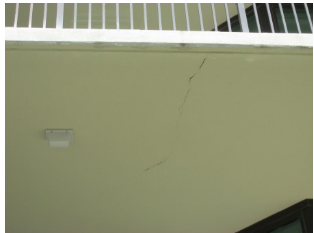
Crack at balcony underside
