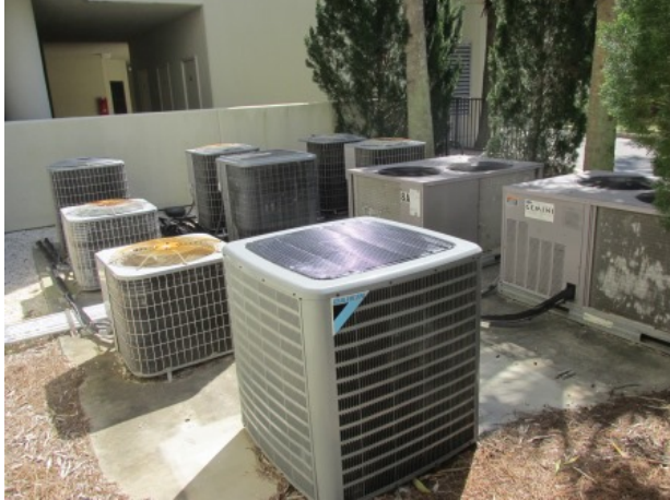
Split system condensing units
