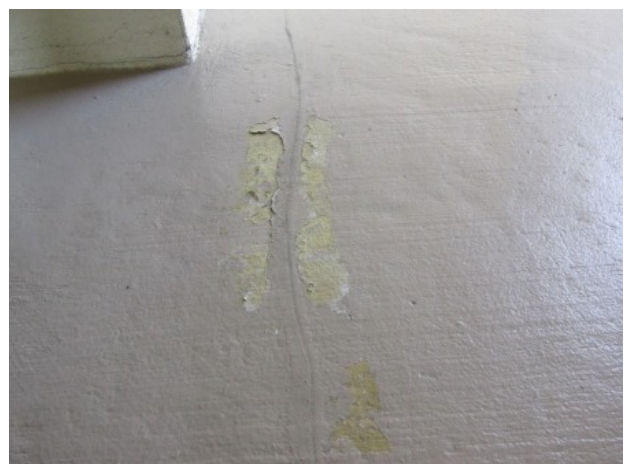
Breezeway crack and finish deterioration
