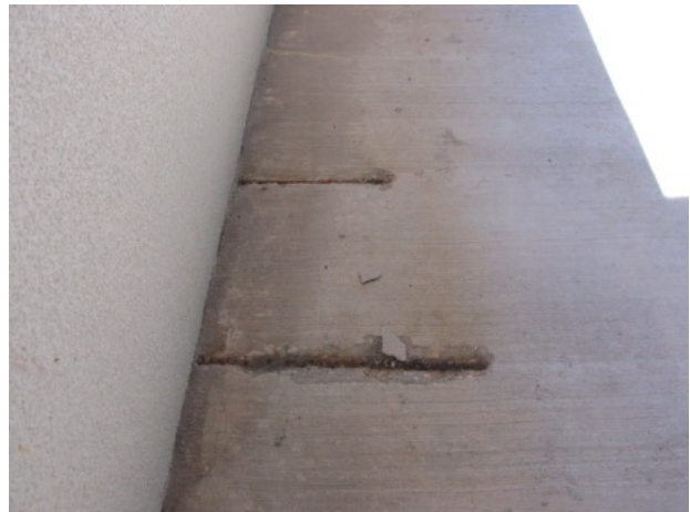
Exposed reinforcement on driving surface
