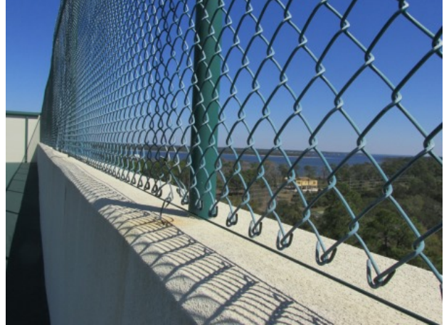
Fence webbing detached from post
