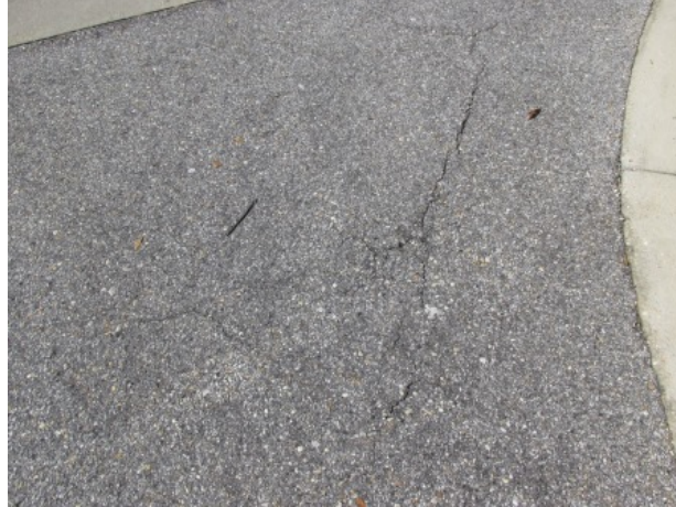
Minor asphalt pavement cracks
