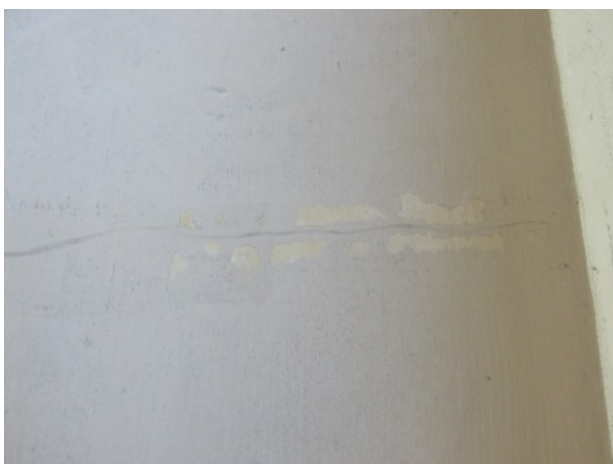
Breezeway crack and finish deterioration
