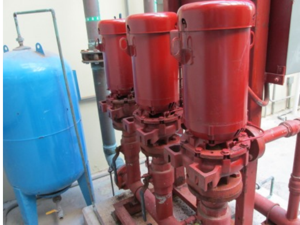
Domestic water pumps
