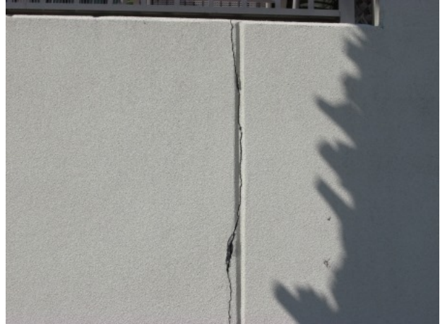
Retaining wall crack
