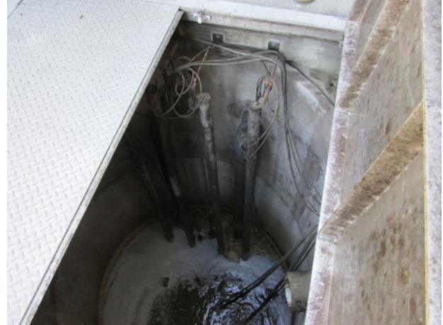
Lift station rails
