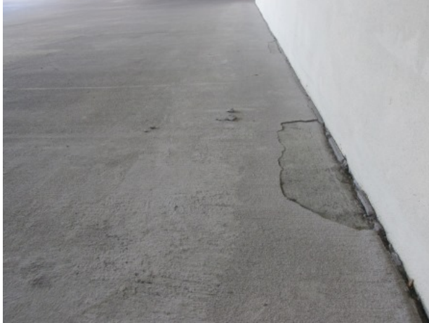
Chipped concrete at the driving surface
