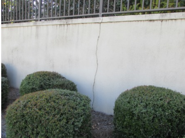
Retaining wall crack
