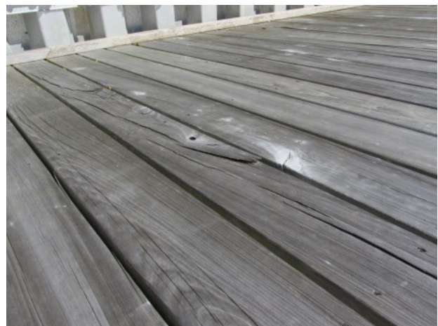
Weathered deck boards
