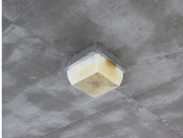
Typical light fixture
