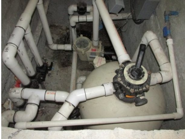
Pump and filter
