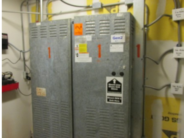
Typical elevator equipment
