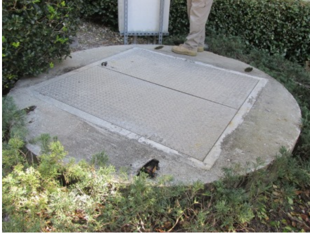
Lift station top
