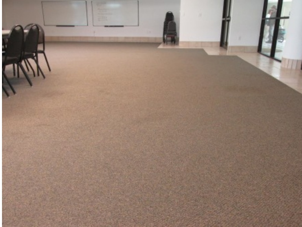
Meeting room carpet – note stains
