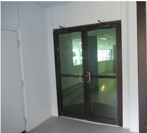
Common area doors
