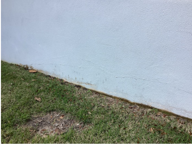
Wall stucco cracks
