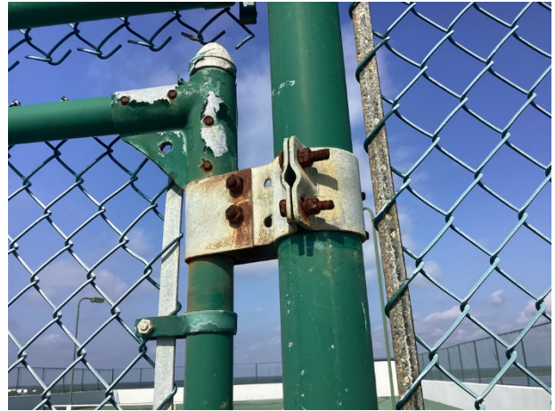
Fence post rust
