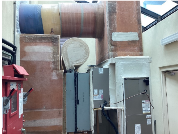
Pool dehumidification unit
