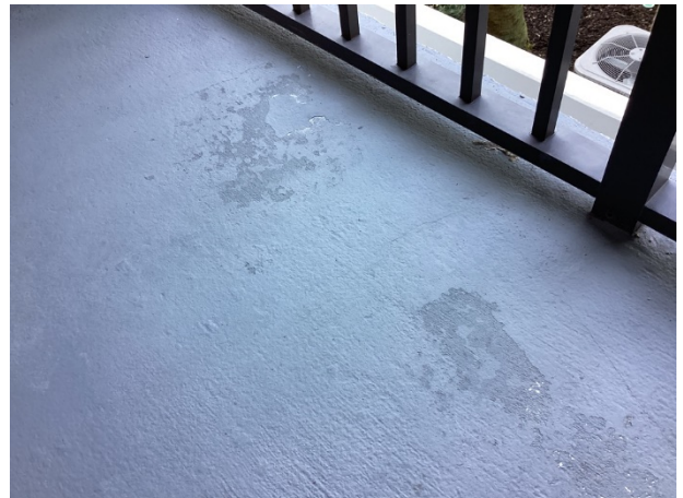
Evidence of isolated chipped coatings
