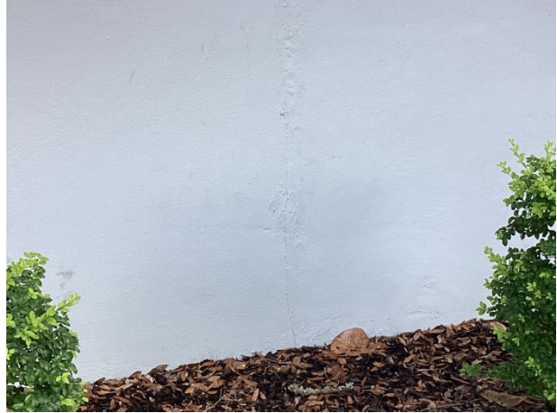
Wall stucco cracks
