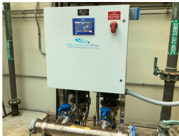
Domestic water pumps
