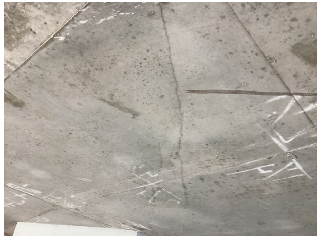
Concrete cracks at ceiling
