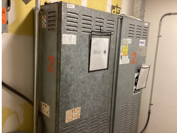
Traction elevator controls
