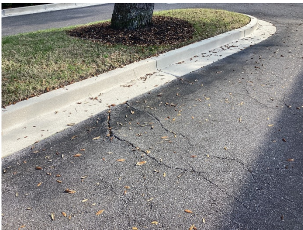
Pavement cracks due to tree root uplift
