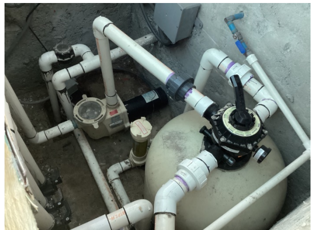
Pool mechanical equipment for fountains
