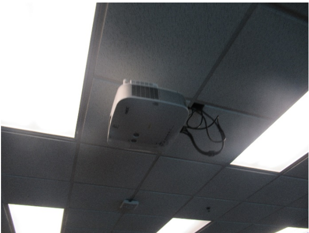
Overview of audio and visual equipment
