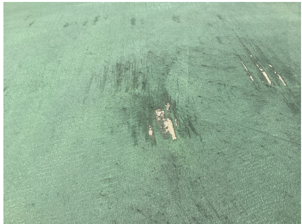
Chipped waterproof coatings
