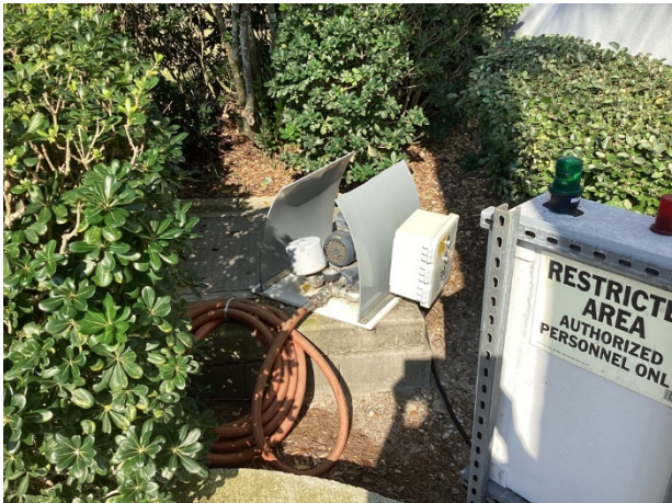
Lift station pump
