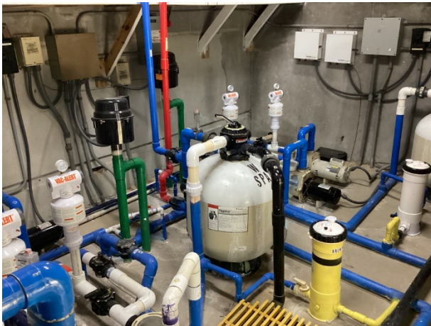
Pool mechanical equipment
