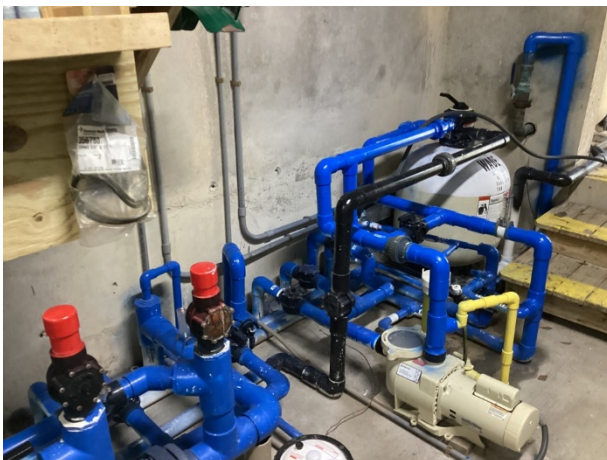
Pool mechanical equipment
